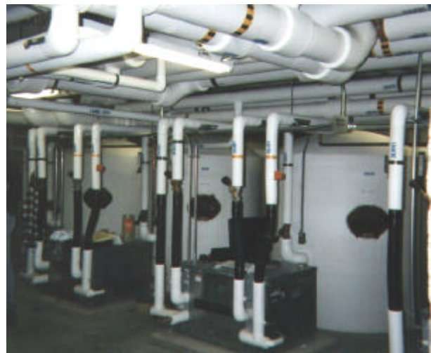
Figure 5. Water Heating System Heat Pumps and Storage Tanks
